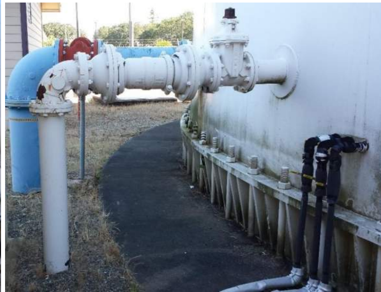
Exterior Anchors and Piping
