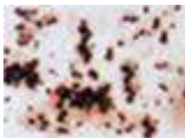
Figure 9 Society for Protective Coatings (SSPC)-Vis 2 Rust Grade 4 (End of Useful Coating Life)
