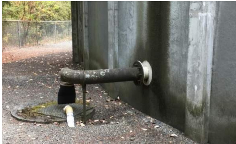
Exterior Staining and Dampness
