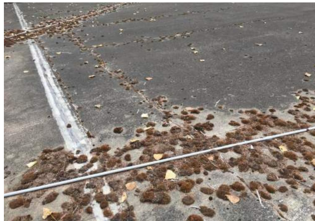
Moss on Roof
