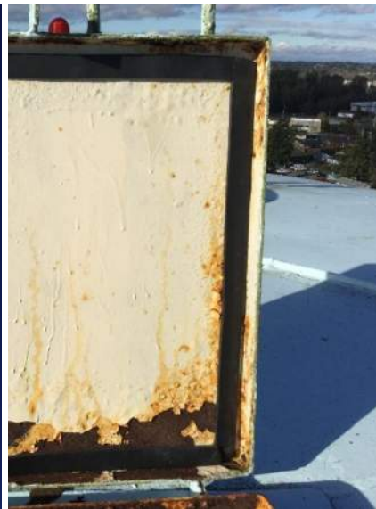
Corrosion at Access
