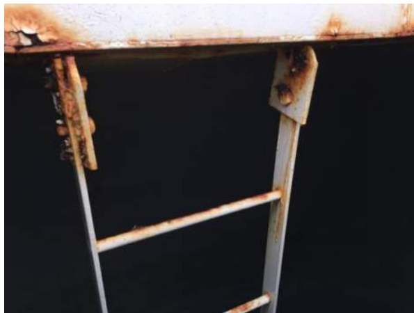
Corrosion at Interior Ladder
