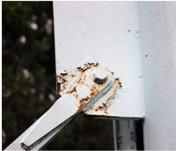
Brace Connection Corrosion
