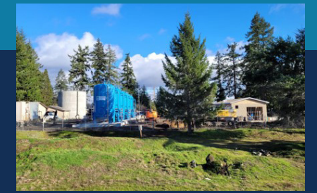
Scotts Wellfield Treatment Project
