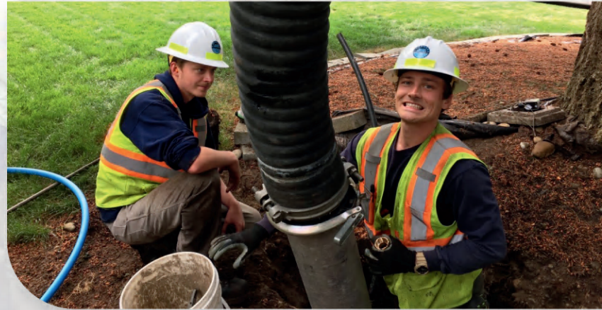
(Above) Kyle and Tyler use rented vac truck to free meter boxes of tree roots without having to remove trees
