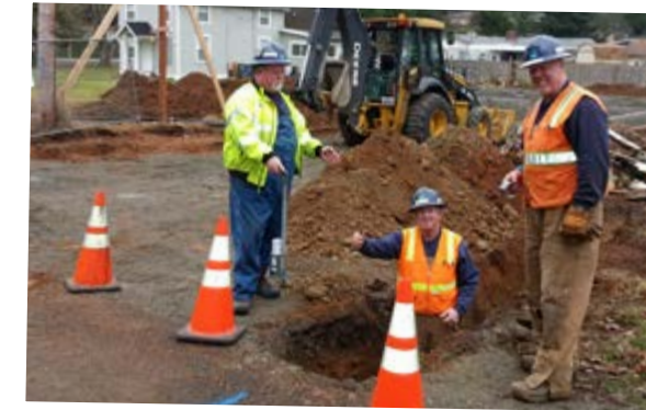
Dick, Rich, and Sam install a new water service line for a customer on Wildwood Avenue
