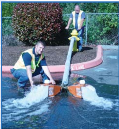
Flushing our system regularly helps keep your water clean and safe.
