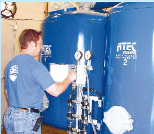
Monitoring Filter System in New Filtration Plant
