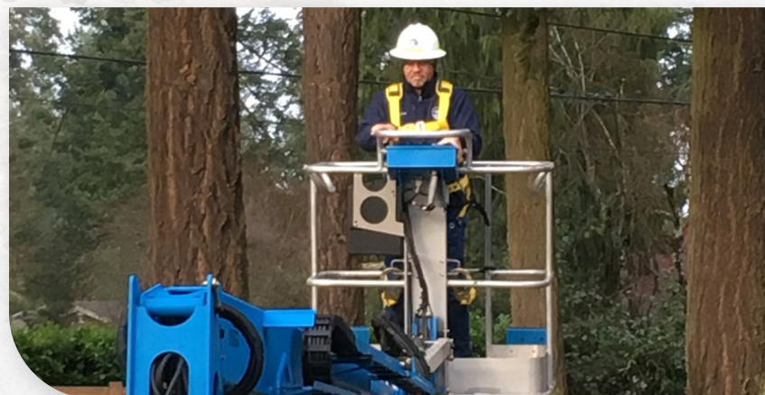
(Above) Bobby using manlift to change bulbs in yard lights and check security cameras
