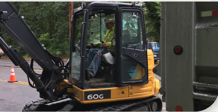
(Above) Eric uses a mini-excavator to load spoils into a dump truck
