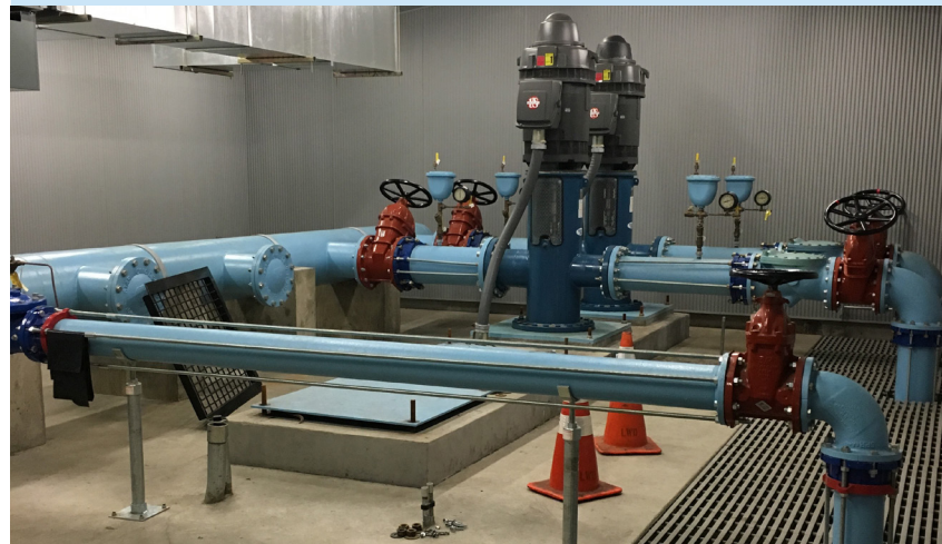
Existing Wholesale Booster Station
