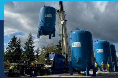
GAC Filter Vessels for Scotts Well Treatment Project
