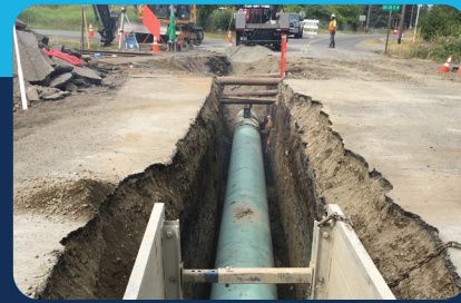
The Water Connection to Spanaway Water
