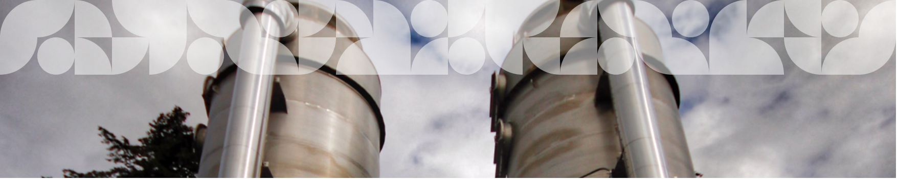
(Above) Twin stainless steel stripping towers at Ponders Wellsite
