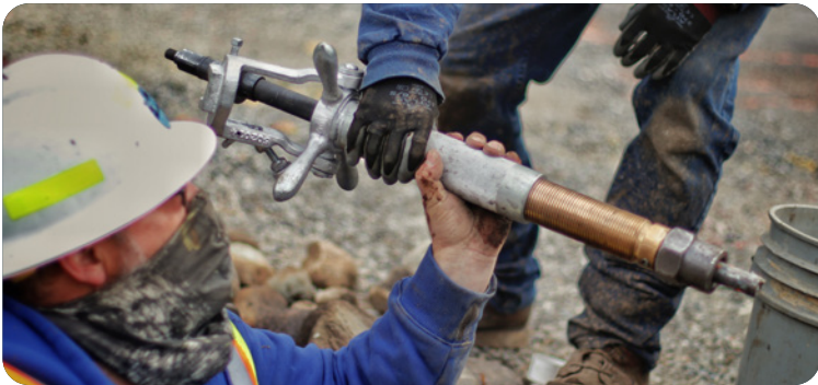
(Top) Eric & Clark repair hydrant (Middle) Chris takes GIS shot (Bottom) Rod taps a water main
