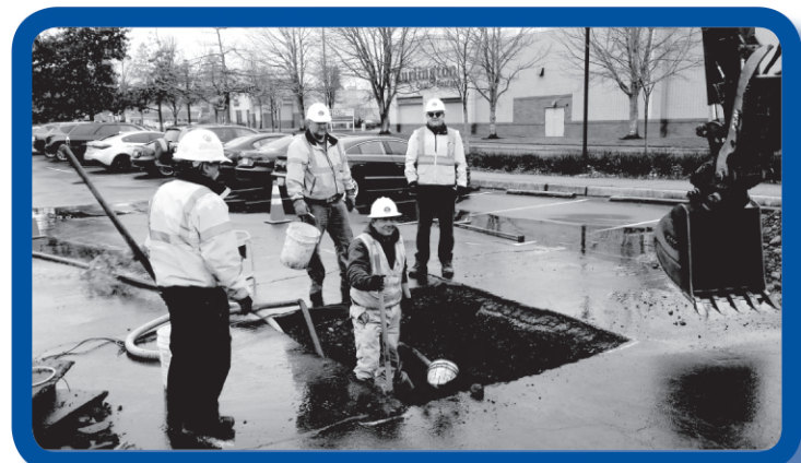
Leak detection helped our LWD team find and fix a main break in Lakewood Towne Center.
