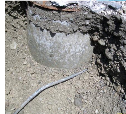
Service line bent
