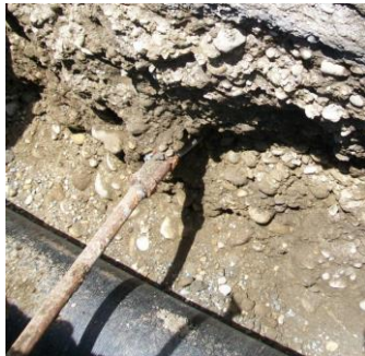
Service line leak
