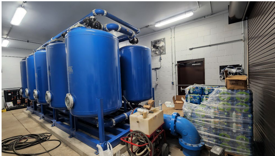
G-3 Well Iron/Manganese Treatment Filters
