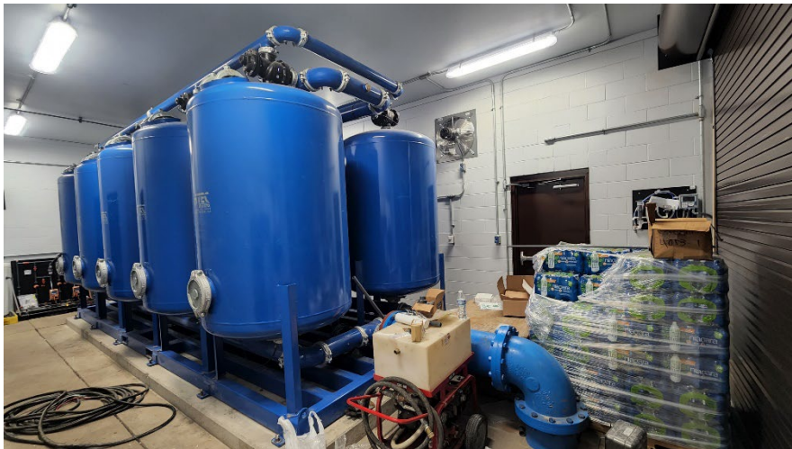
G-3 Well Iron/Manganese Treatment Filters
