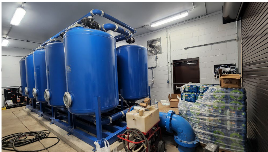
G-3 Well Iron/Manganese Treatment Filters
