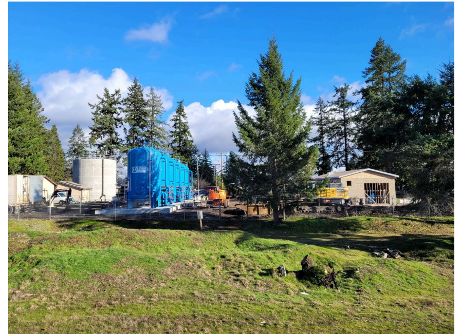
Completed installation of GAC System
