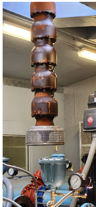
Newly installed screen on pump inlet
